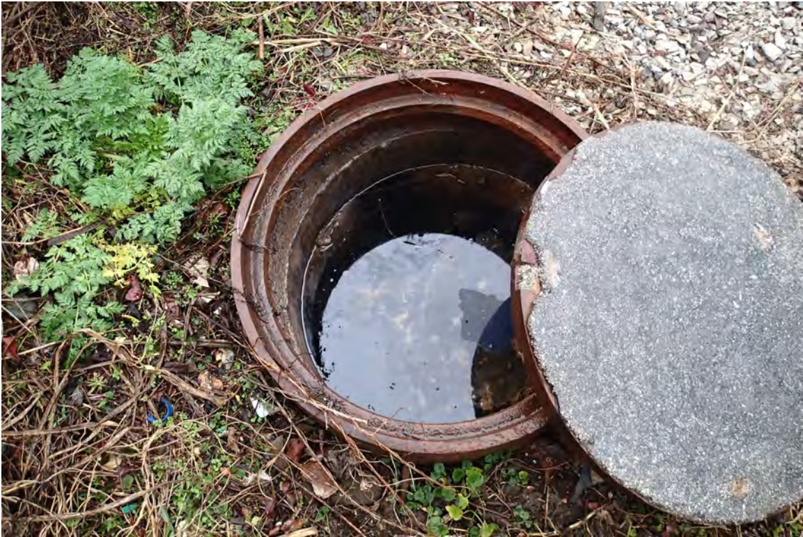
Photo 47: Storage tank opening for runoff water from compactor pad.
