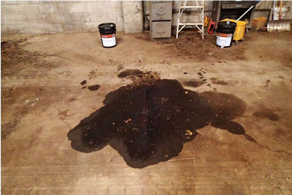
Photo 9: Oil spilled on building floor.
