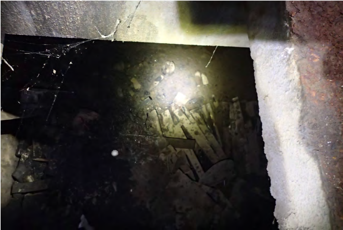
Photo 17: Debris in confined space area under building floor.
