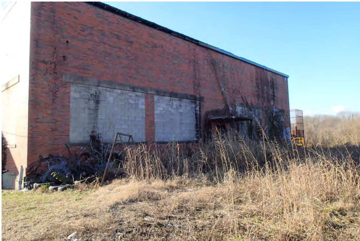
Photo 6: Fascia board missing on north side of building.
