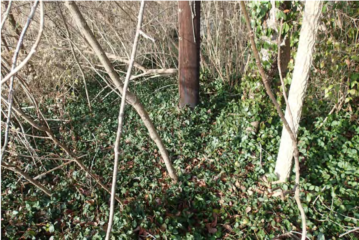
Photo 33: Base of power pole near shooting range. No evidence of transformer leaking oil.
