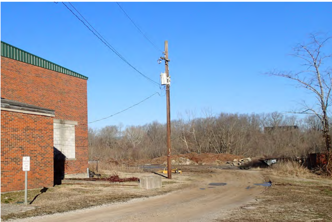
Photo 34: Power company confirmed this transformer is PCB free.
