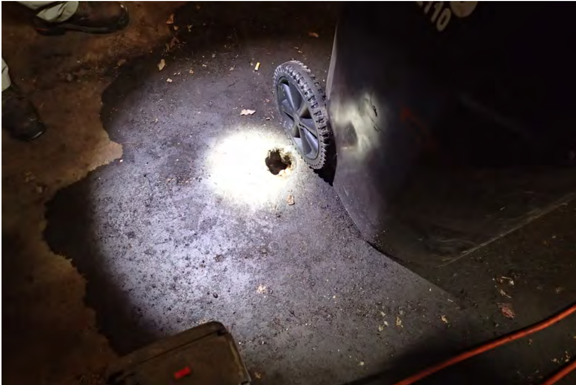
Photo 15: Oil spilled inside building around floor penetration.
