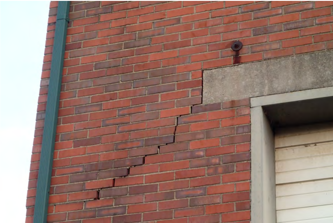
Photo 5: Building Settlement issues on south side of building.
